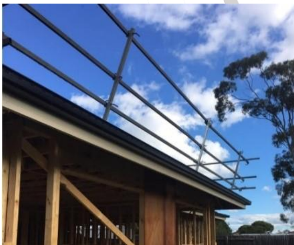
Guard Rail Protection
